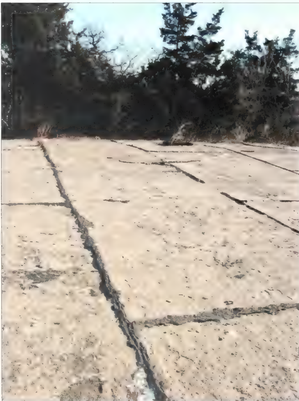
Figure 5.70. Close-up view of existing concrete terreplein, Battery Granger. Existing conditions indicate that joints between concrete panels were once sealed with bituminous material. With the passage of time, this sealant material requires maintenance (Olmsted Center, January 2009).
